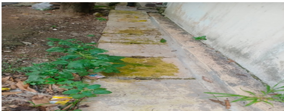
Figure 2. Condition of existing drainage channels
